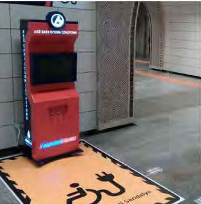
Image C.21 Free standing electric wheelchair charging station in the metro station, Istanbul, Turkey. Source: http://www.dailysabah.com/nation/2014/12/11/battery-charging-units-for-wheelchairs-in-istanbul-metro-stations
