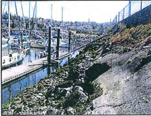
Photo 1. Vegetation along the steep shoreline bank is limited to areas with cracks in the concrete or voids between riprap rocks (Photo: AES, 6/16/2015).
