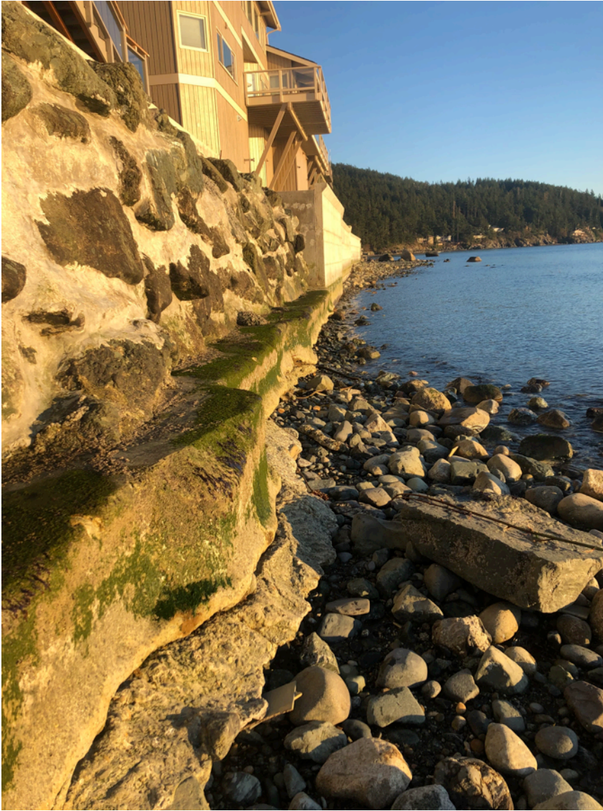
Signs of undercutting, debris on the beach and a new, permitted wall to the east.
