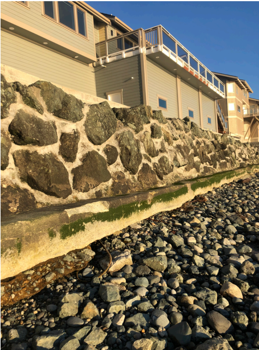
Signs of undercutting.
