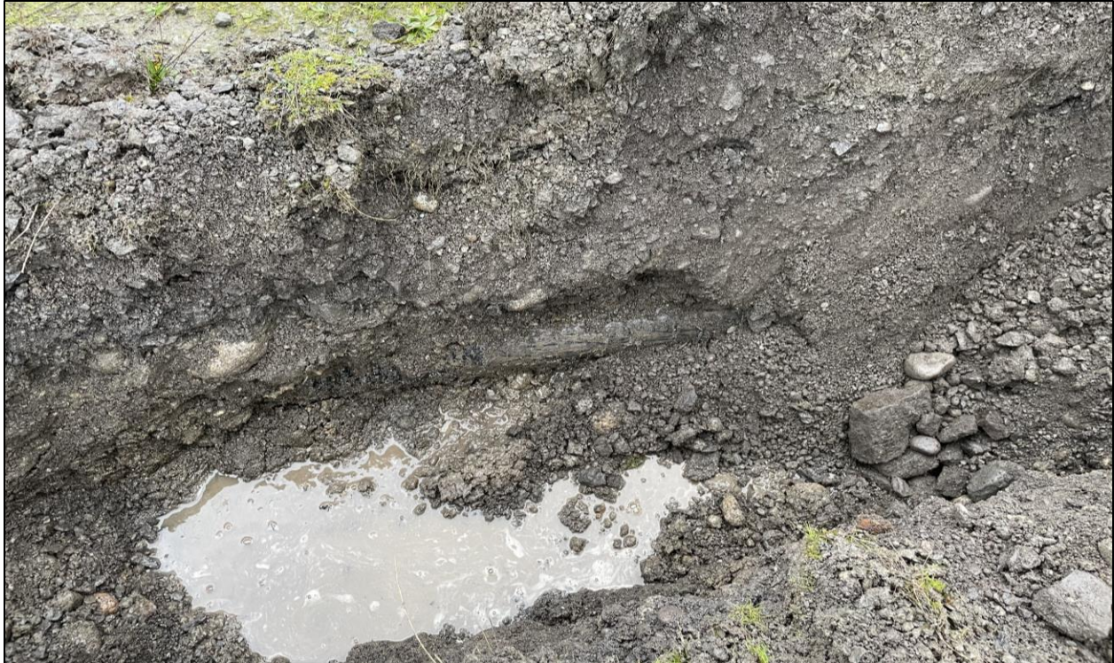
Photo 9. Example of abandoned utility line encountered during testing.
