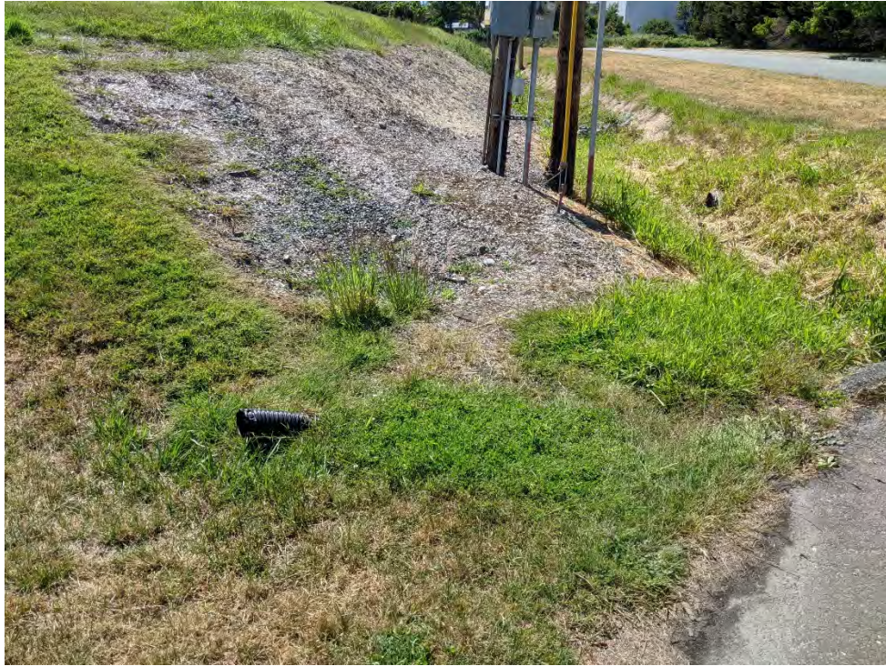
Image 5: Drainage at the SW corner of T Ave & 6 th St, looking West
