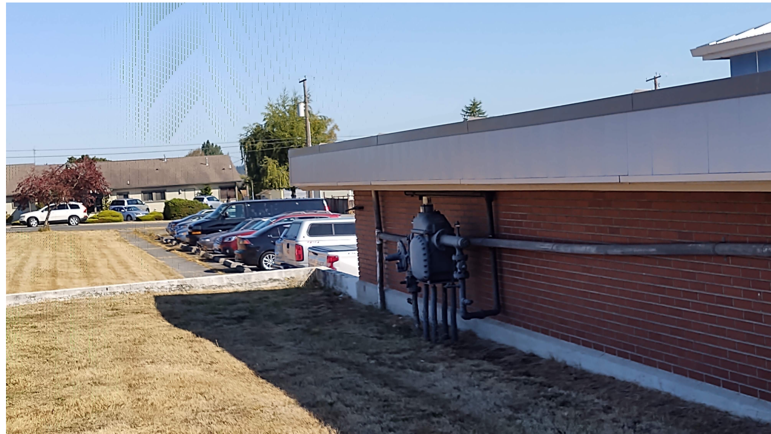
IMAGE P: EXISTING METER AND GAS LINE. LOOKING AT NORTH EAST CORNER, EXTERIOR OF VAULT, ROOM 17.
