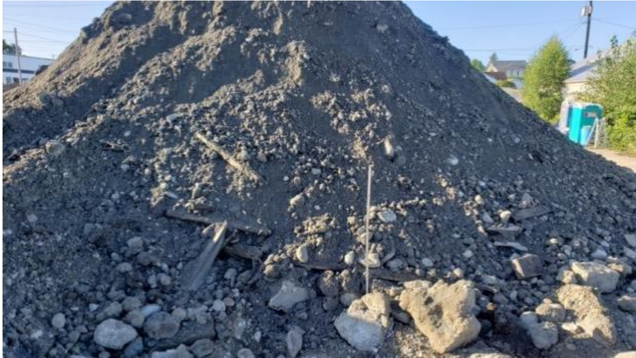
Figure 12. Example of timber in spoils.
