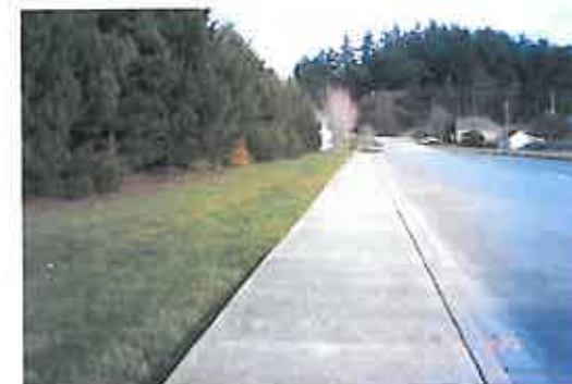
Figure 30. Existing Sidewalk on 6th Street
