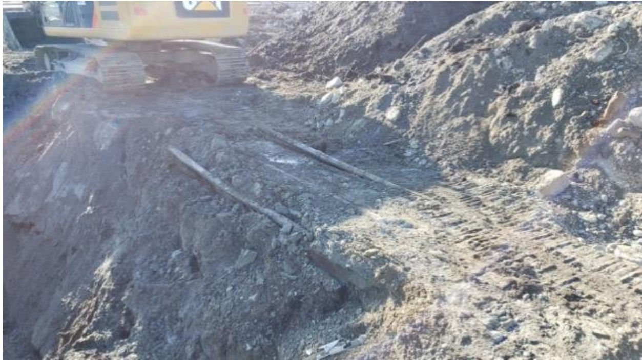
Figure 14. Product lines / pipe platform, facing ESE from driveway on Western edge of project.
