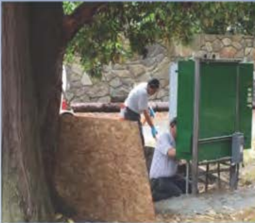
Odi Flores and Jordan Davis, making upgrades to control panel components as part of the Fiber Telemetry upgrade
