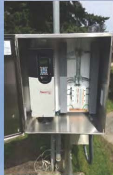
Inside View of the Control Panel
