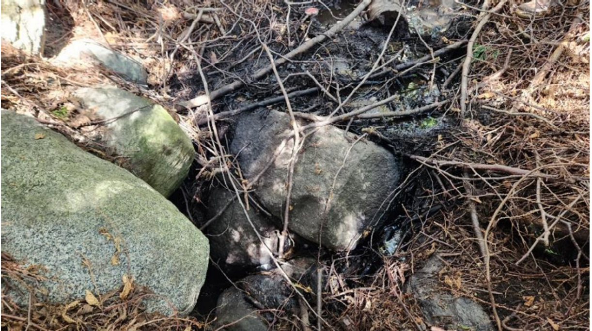
Failed roadway embankment blocking culvert inlet at Clyde Way
