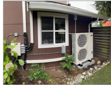
Heat pump installation at residence in Washington State.
