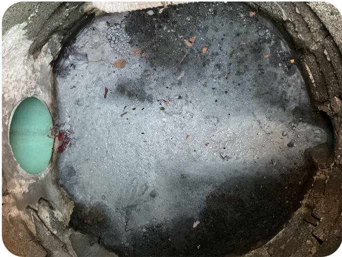
Concrete found in catch basin during an inspection
