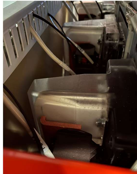
Photos of Pump #4 inverter replaced last year
