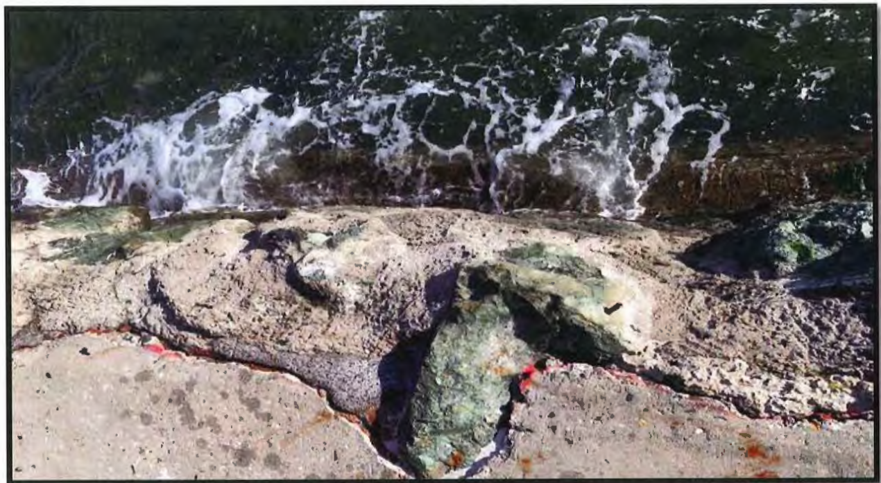
Schutzler Existing Bulkhead (during high-tide)
