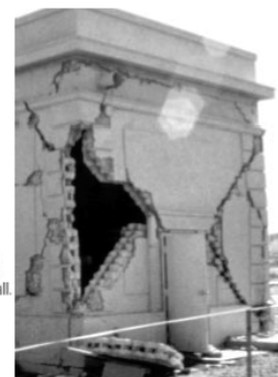
Damaged masonry wall
