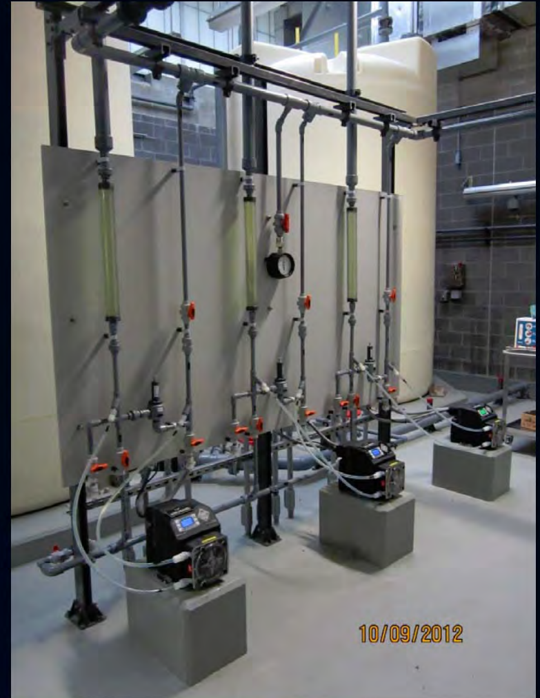
City of Bremerton's hypochlorite feed system
