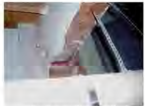
Beam connection to wall with no fire-blocking
