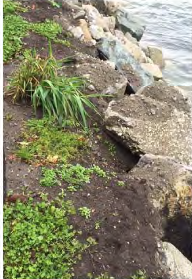
Photo 7. New bare soil is already eroding and washing away on the waterside edge of the trail. Cover with erosion jute and immediately plant soil binding ground. Place arborist chips over the jute and around the plants, but not against the stems of plants. Additional rip rap should also be considered to protect loose soils.
