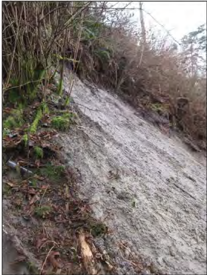
Photograph 4: Shallow recent slide along the bluff above the trail.
