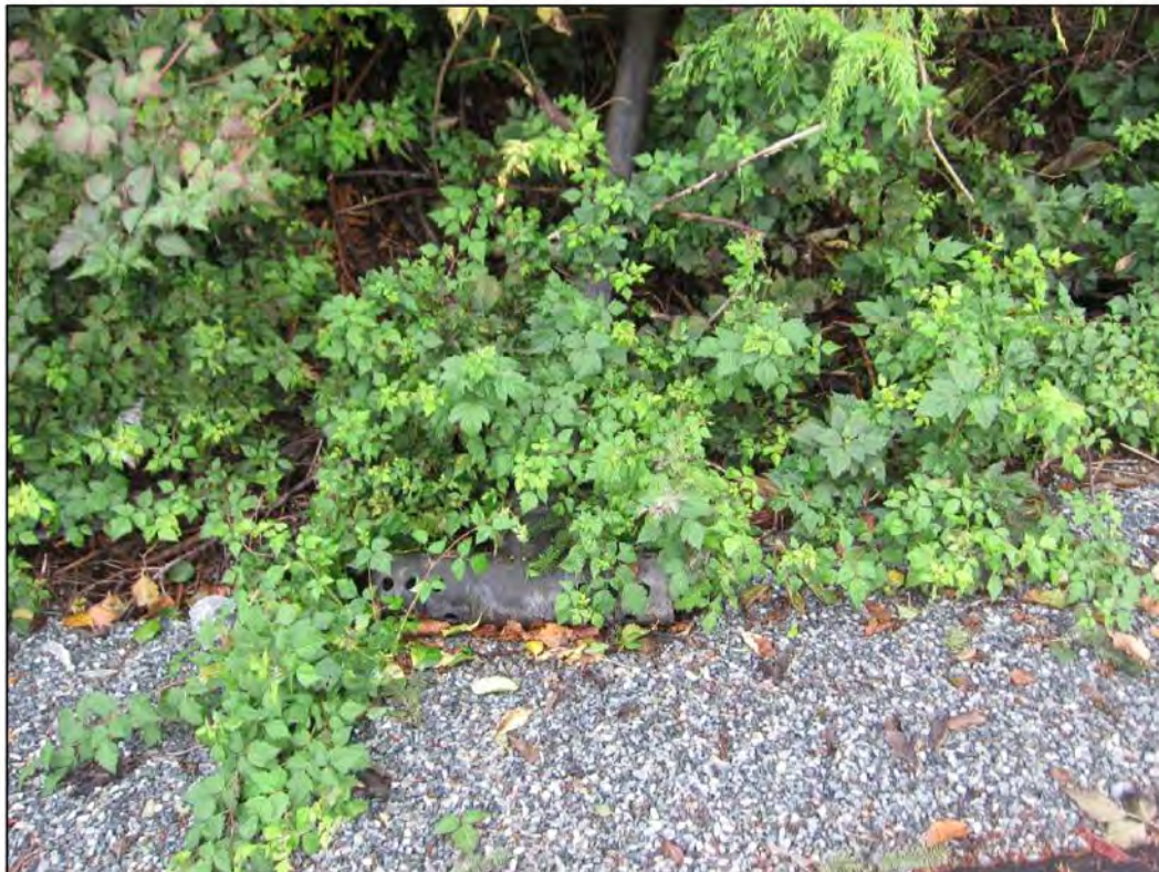
Photograph 3: Small HDPE pipe with T energy dissipater.
