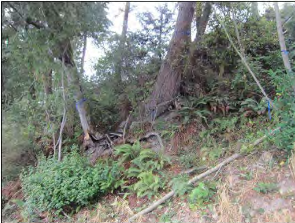
Photograph 5: Several trees that have undermined roots that could lead to failure and further slope destabilization.
