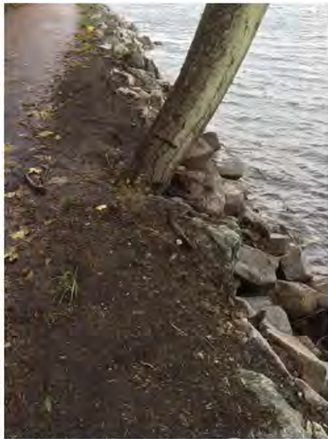
Photo 2. Newly placed and exposed soil between the trail and shoreline rip rap is especially vulnerable to erosion from rainfall, storm water runoff and ocean splash. Proper measures must be taken to reduce potential erosion and hasten the establishment of strong vegetation cover.
