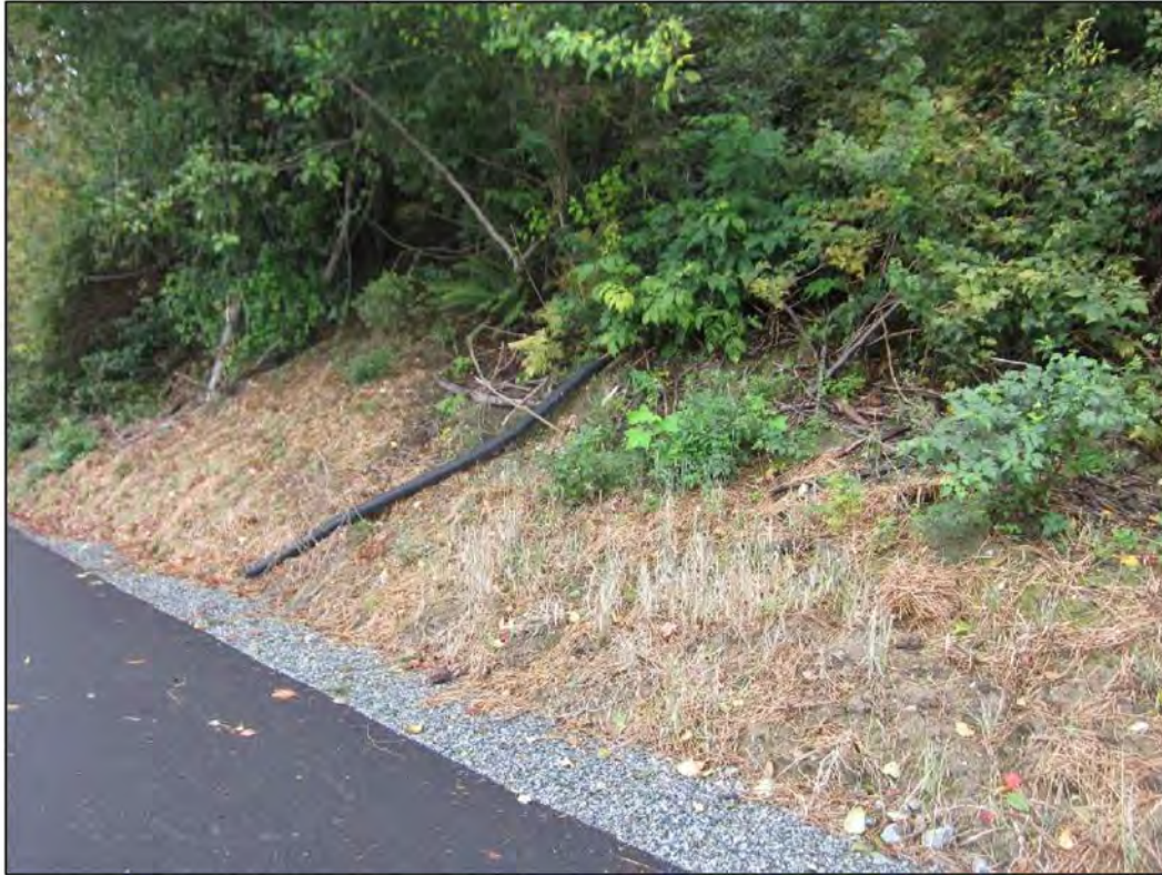
Photograph 2: Light duty corrugated pipe with no energy dissipation.
