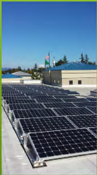
Police Station 15.95 solar array
