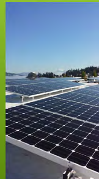
City Hall 21.45 solar array
