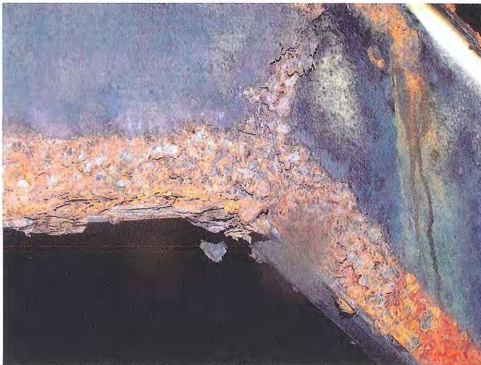
FIGURE 22 Significant Corrosion at a W10 Beam
