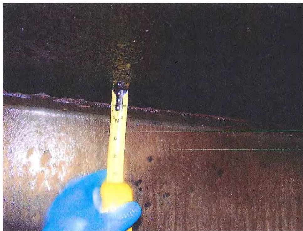
FIGURE 30 Example of Gap Between Top of Beam and Underside of Roof Plate
