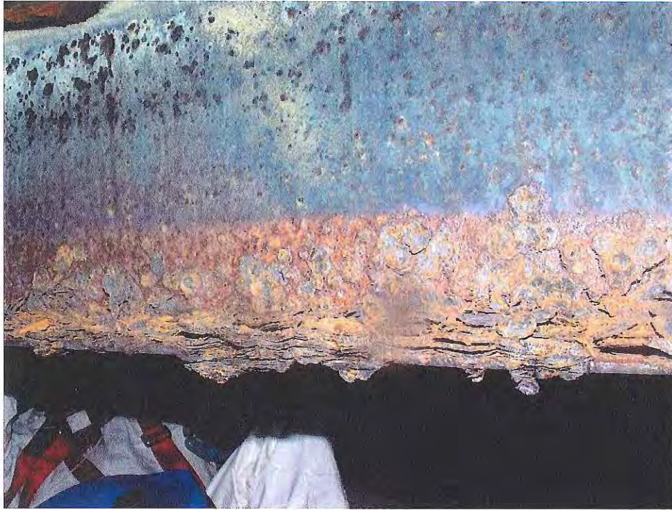
FIGURE 21 Significant Corrosion at a W10 Beam
