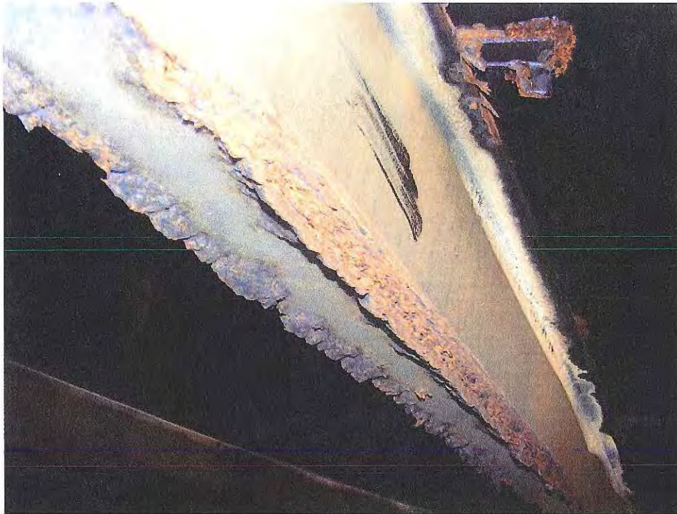
FIGURE 27 Significant Bottom Flange Corrosion of a W10 Beam
