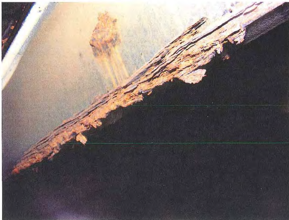
FIGURE 24 Significant Corrosion at a W10 Beam
