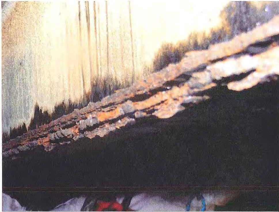
FIGURE 25 Significant Corrosion at a W10 Beam
