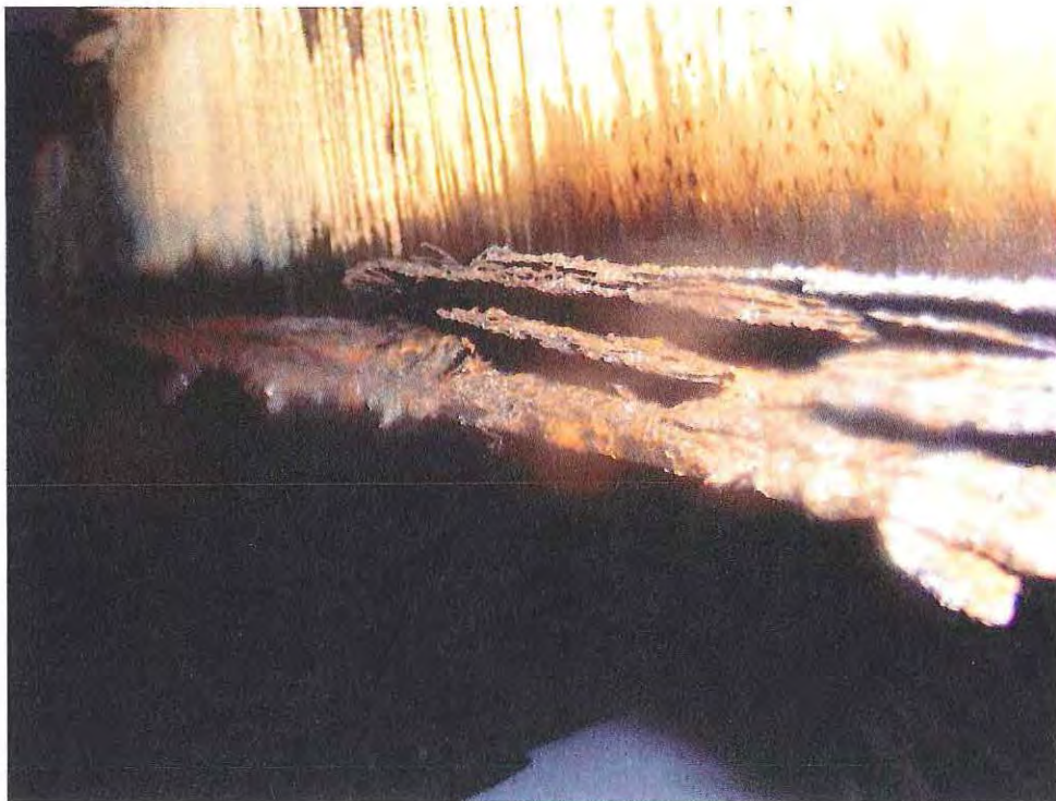
FIGURE 16 Bottom Flange of a W10 Beam with Rust "Laminations"
