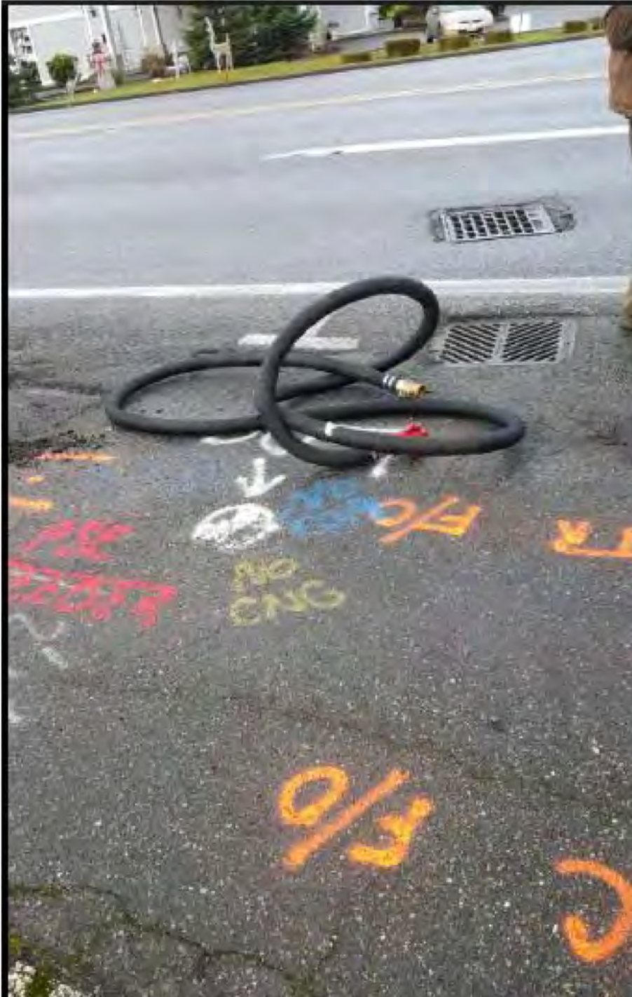
Photo 4: Utility conflicts and limited space that did not allow for boring opportunities at Sharpes Corner.
