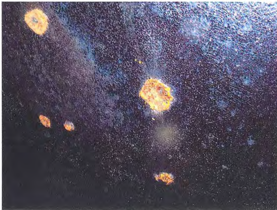
FIGURE 36 Example of Pitting on Underside of Roof Plate
