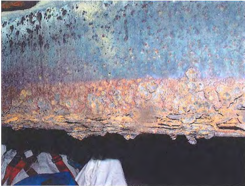
FIGURE 21 Significant Corrosion at a W10 Beam
