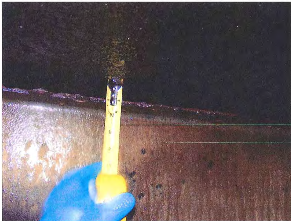
FIGURE 30 Example of Gap Between Top of Beam and Underside of Roof Plate
