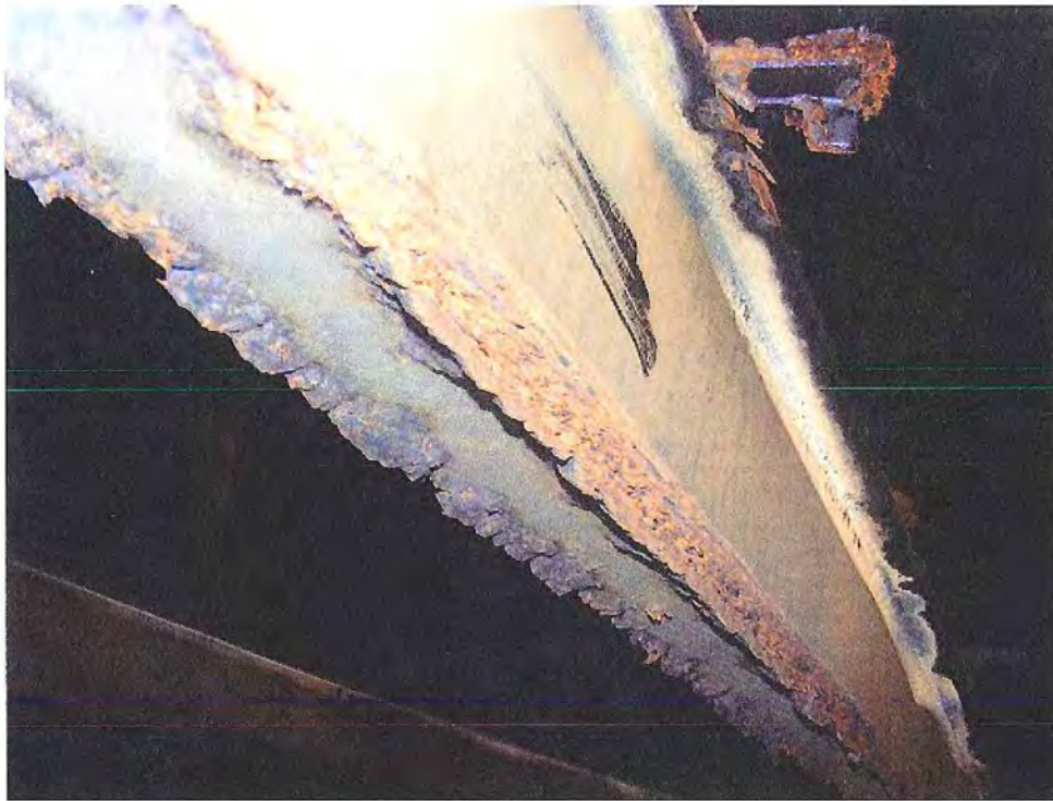
FIGURE 27 Significant Bottom Flange Corrosion of a W10 Beam
