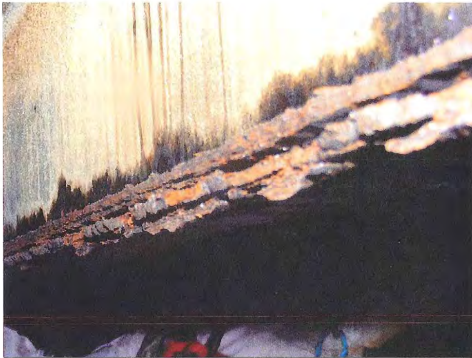
FIGURE 25 Significant Corrosion at a W10 Beam
