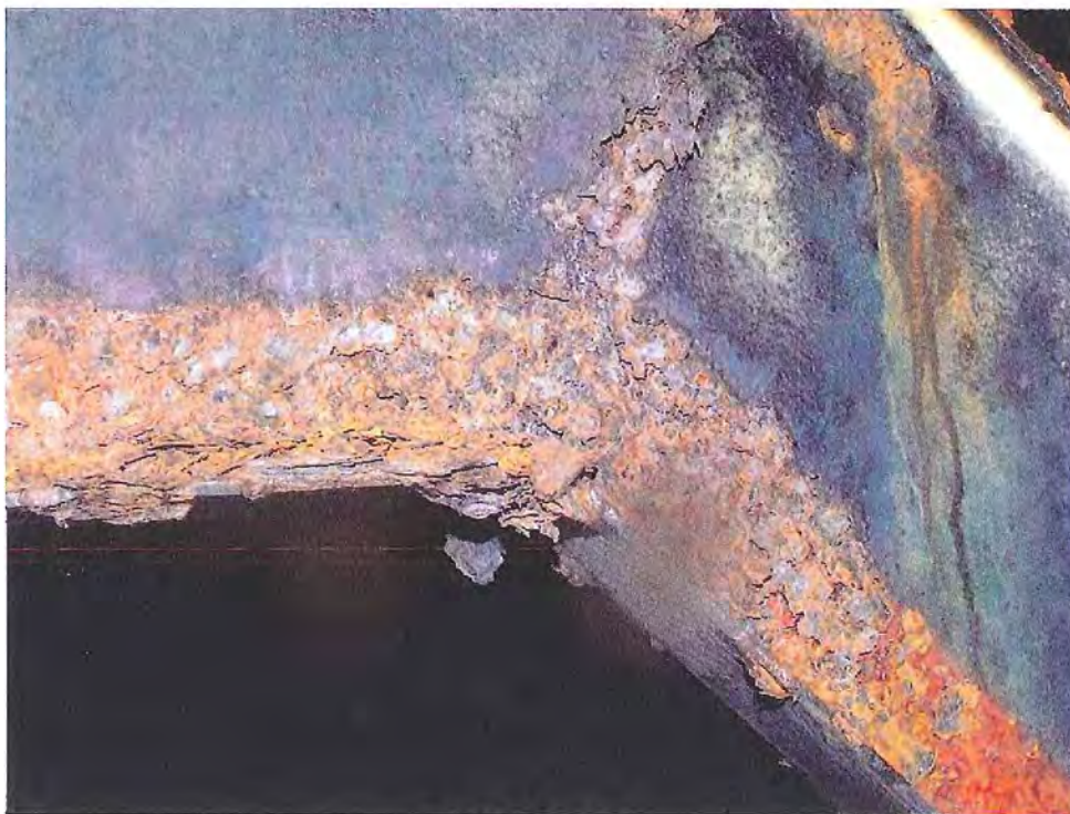
FIGURE 22 Significant Corrosion at a W10 Beam
