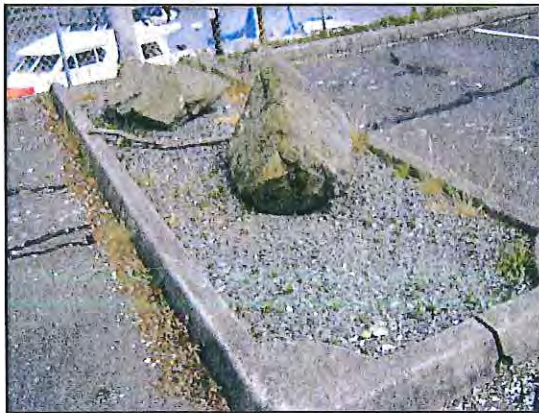
Photo 9. Vegetation is lacking in planter area L5. Three snowberry shrubs and 2 kinnikinnick ground cover plants are proposed for installation in this area. Topsoil and mulch will replace existing gravel (Photo: AES, 5/11/2016).
